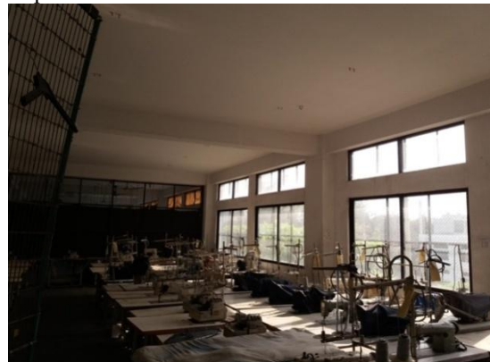
Figure: Opening at southwest wall
